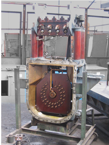
Tap changer inside a transformer
